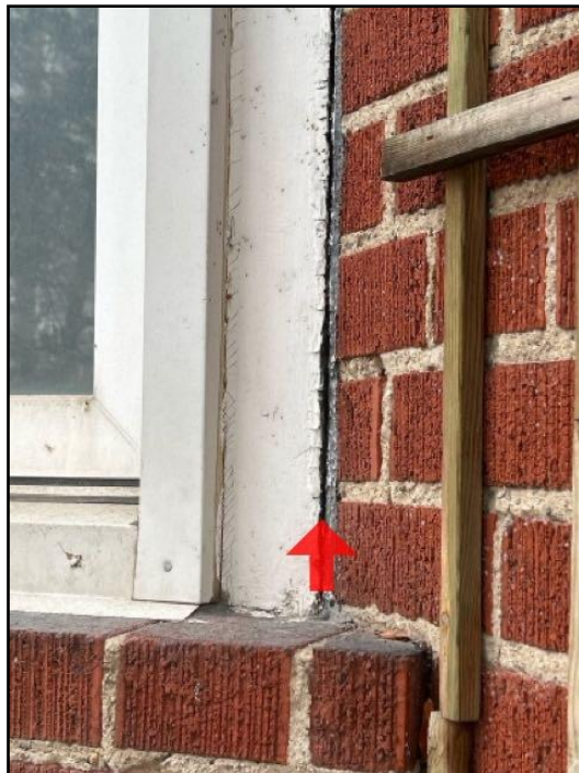
Caulking missing, loose or deteriorated
