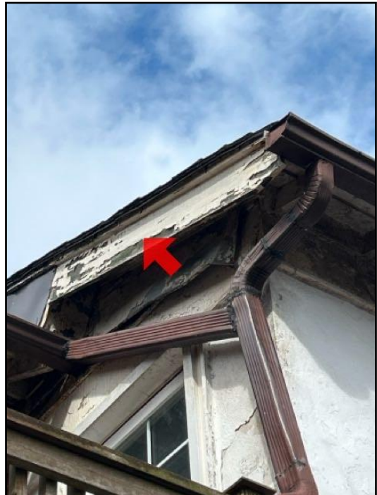
Paint - deteriorated / missing
