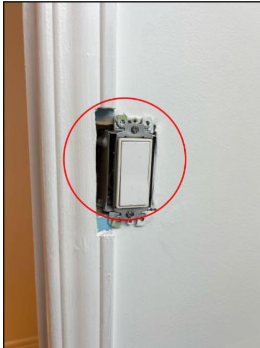
Missing cover plate
