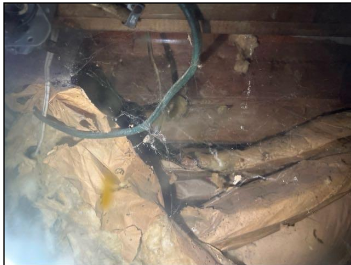
Loose, missing insulation
