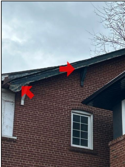
Paint - deteriorated / missing
