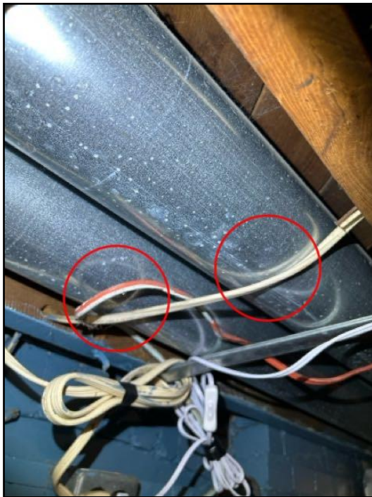
Too close to/touching duct, pipe, vent or...
