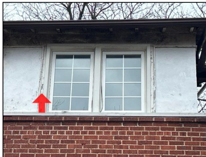
Paint or stain needed
