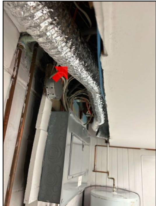
Duct run too long
