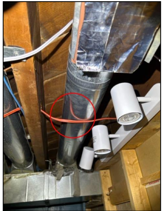
Too close to/touching duct, pipe, vent or...
