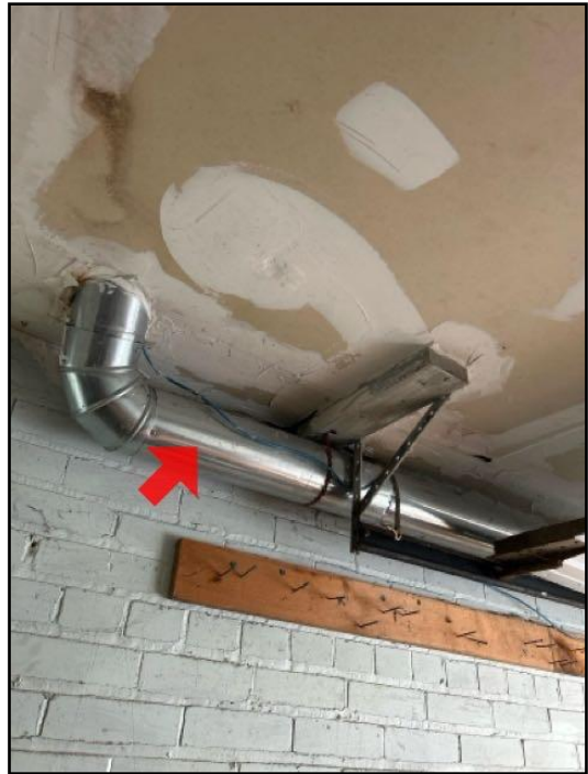
Insulation missing, damaged
