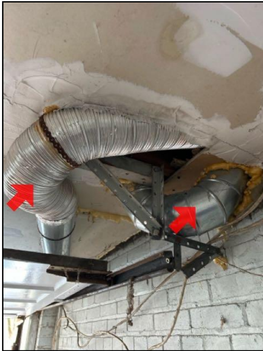
Insulation missing, damaged
