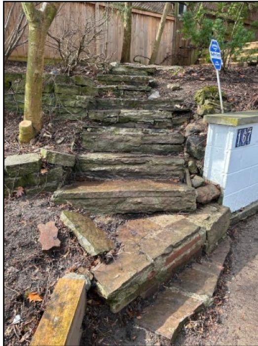
Steps or landings settling or heaving
