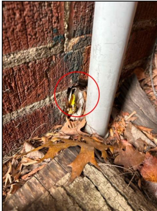
Improperly patched hole
