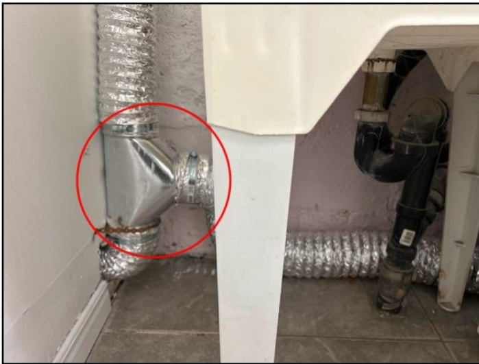
Manifolding of dryer and bathroom exhaust
