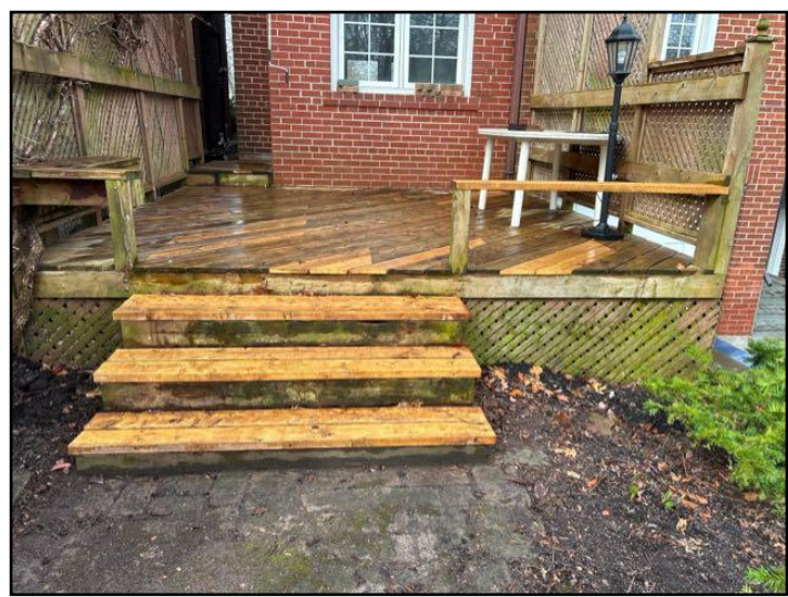
Guard and handrail issues
