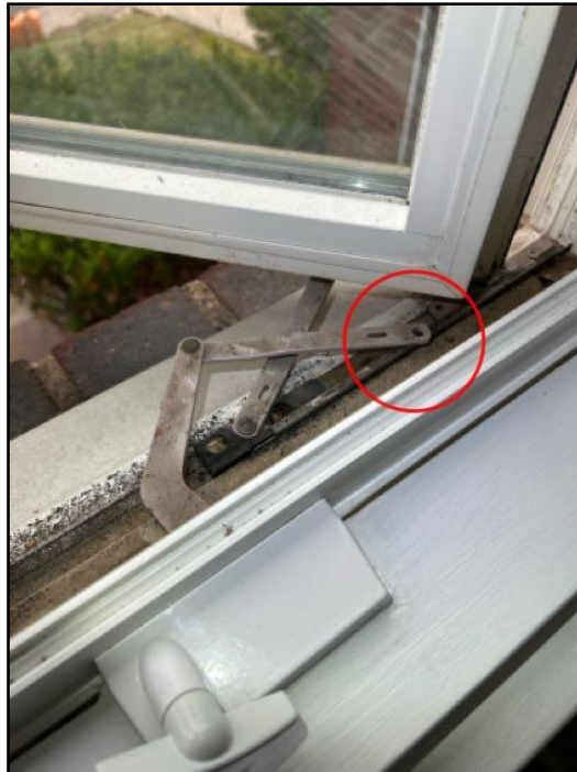
Broken - loose control arm
